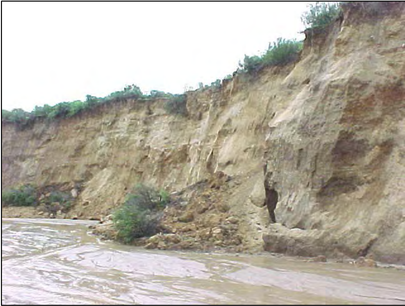
FIGURE 1-5C An urban stream, the Lower Oso Creek in Orange County, California, following a storm event. Oso Creek was formerly an ephemeral stream, but heavy development in the contributing watershed has created perennial flow—stormwater flow during wet weather and minor wastewater discharges and authorized non-stormwater discharges such as landscape irrigation runoff during dry weather. Courtesy of Eric Stein, Southern California Coastal Research Water Project.
