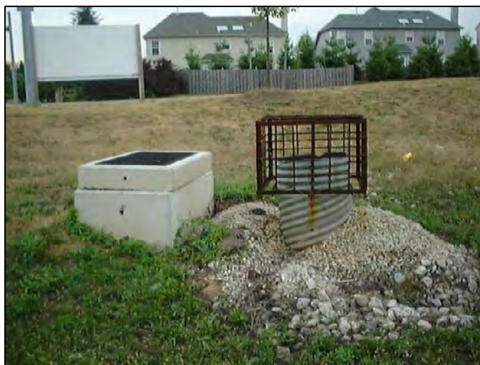
FIGURE 5-8 Sediment filter left in place after construction. SOURCE: Robert Traver, Villanova University.
