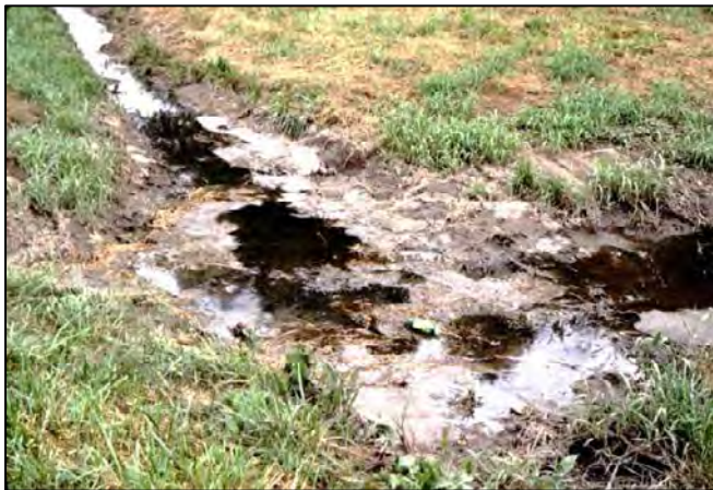
FIGURE 3-32 Failing sanitary sewer, causing upwelling of sewage through soil, and draining to gutter and then to storm drainage system. SOURCE: Robert Pitt, University of Alabama.
