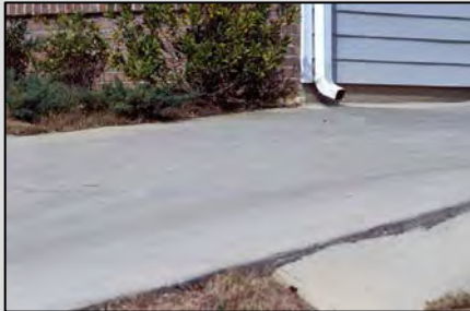
A directly connected roof drain
