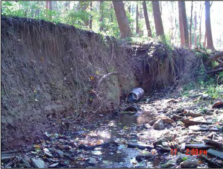
FIGURE 1-5A Headwater tributary in Philadelphia suffering from Urban Stream Syndrome. SOURCE: Courtesy of Chris Crockett, Philadelphia Water Department.
